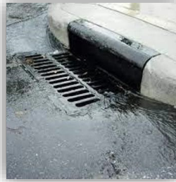
Storm Water Drains
